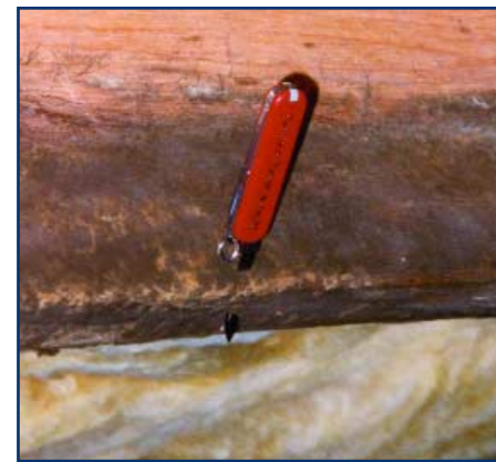
After installation of a powered crawl space ventilation fan, so much water condensed on the floor joists that rot set in and destroyed the lower portion of the joists.
