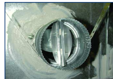
Metal strapping holds this 4 inch (102 mm) diameter supply duct horizontal to ensure proper operation of the butterfly backdraft damper. The balancing damper is visible behind the butterfly damper. The connection to the supply trunk duct is sealed with mastic.
